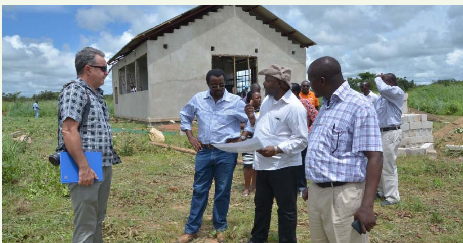
DG Sanginga (with hat) conferring with David Chikoye (second from left), Rod Bishop (leftmost), and Pheneas Ntawuruhunga (rightmost) on the progress of construction of the cassava equipment fabrication facility (at the background) as looks on.
