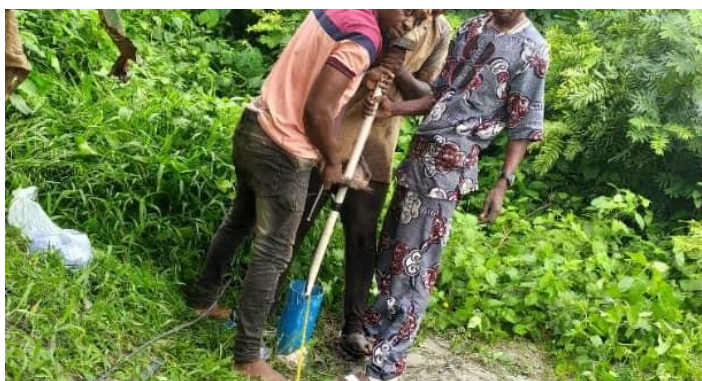
Technicians working on the borehole at Owena Core-trial site (Photo credit: CRIN - Owena)
