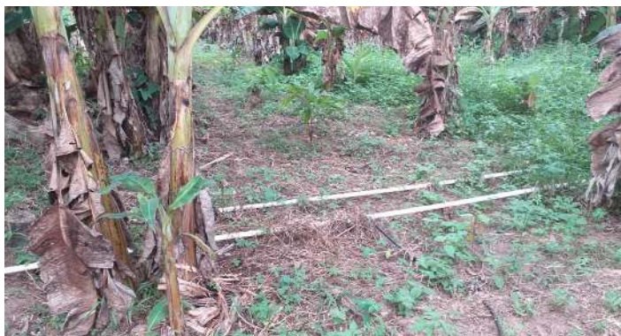
Owena Core trial site showing installed irrigation pipes (Photo credit: CRIN - Owena)
