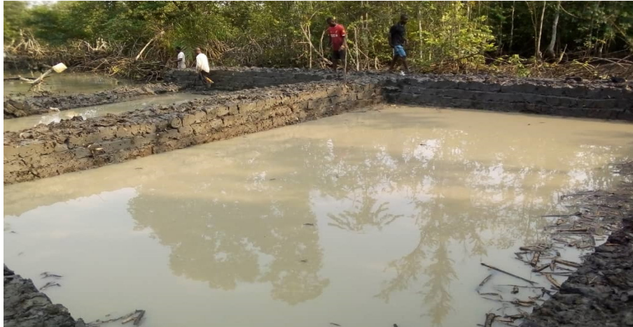
Digging of ponds ongoing at the acquired land by Jemide and partner for aquaculture
