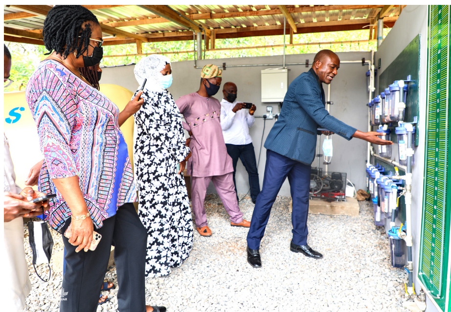
Femi Akeredolu showing NASENI guests how the IITA Biogas plant works.
