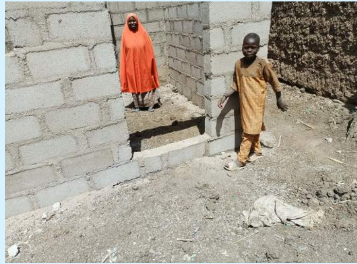
▲ Photo: Mariam Ali' in her new home construction site (Photo Credit FtF-NIAA)
